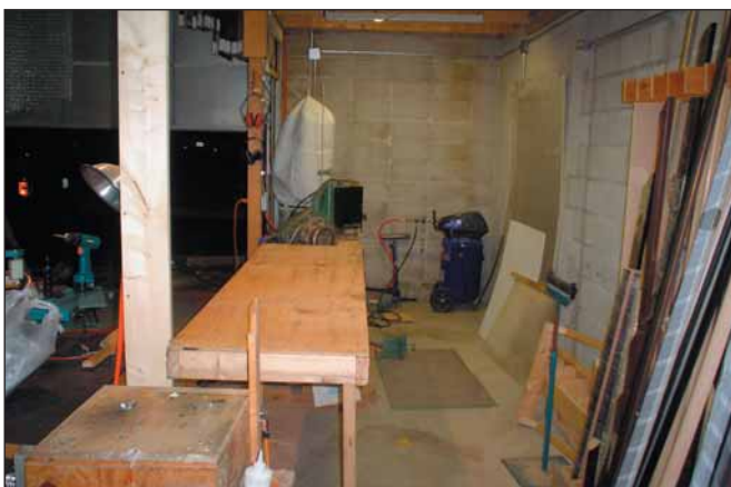
Before (above) and after views looking at the mezzanine area from the lower center of the production area (area C in drawings).
