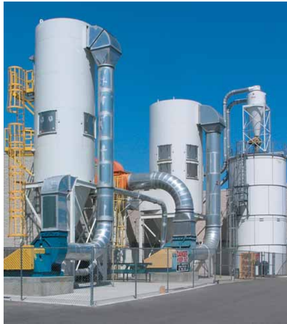
Framerica’s environmental efforts include a state-of-the-art dust collection system that recycles waste to heat the building.
